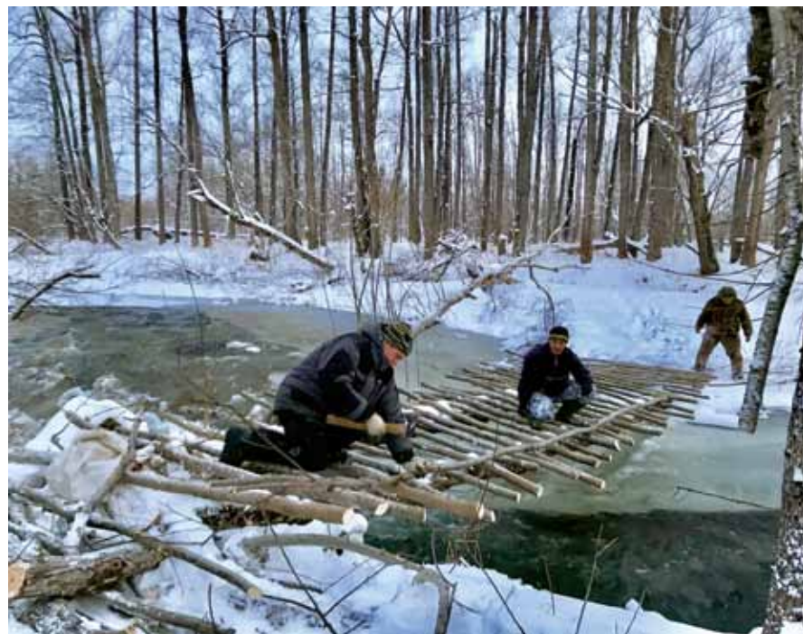
The guides were experts at constructing handmade bridges to get the snowmobiles across streams.
